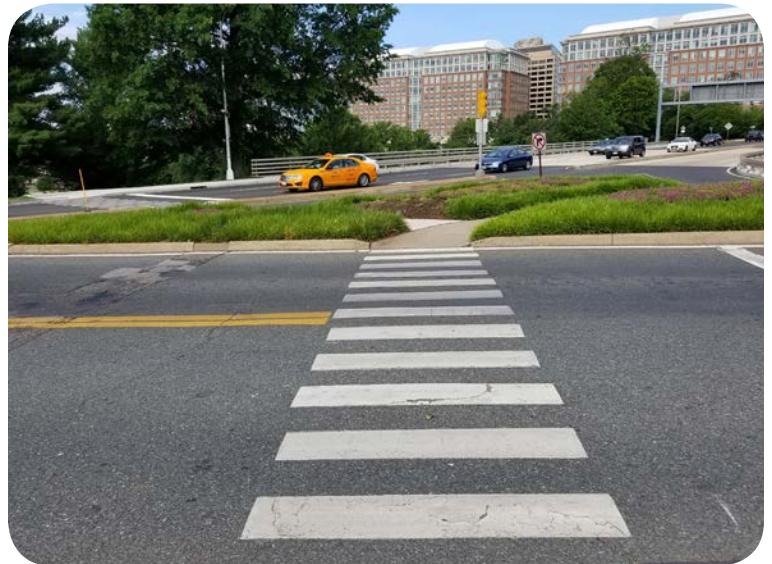
Figure 24 26th Street Bridge intersection lacks legible pedestrian crossing signals.
